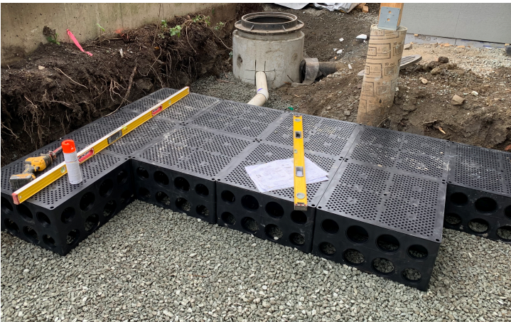
Marino Cell Installation in Victoria, BC
