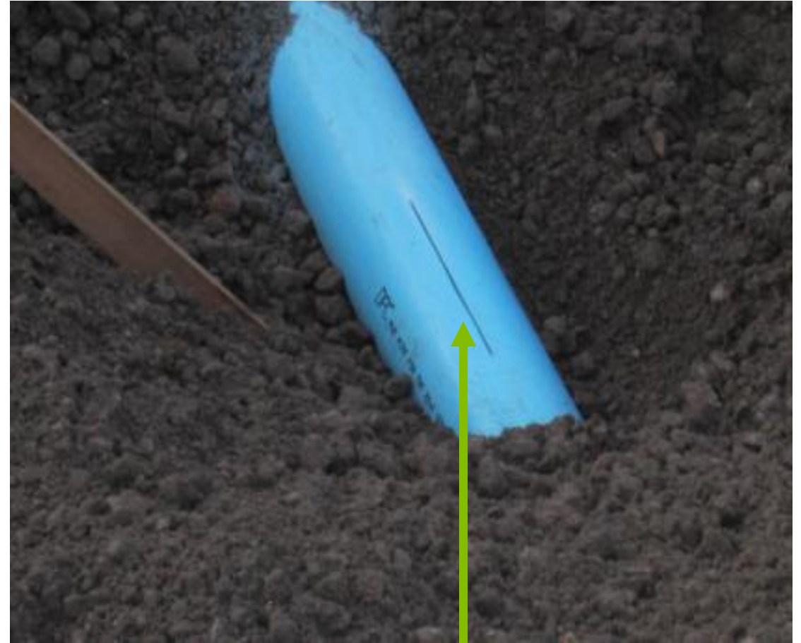
A saw cut was made into the pipe to act like a break in the pipe
