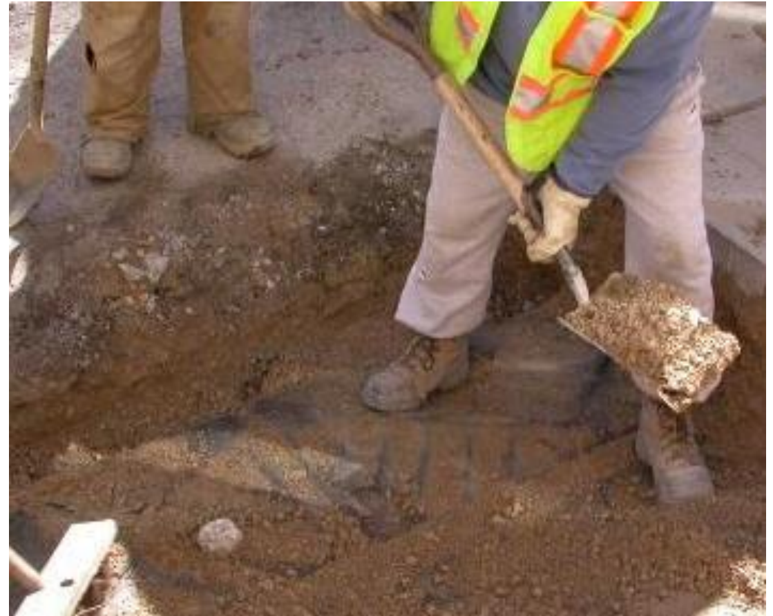
The aggregate base is removed and the fabric covering the decks is cut and removed
