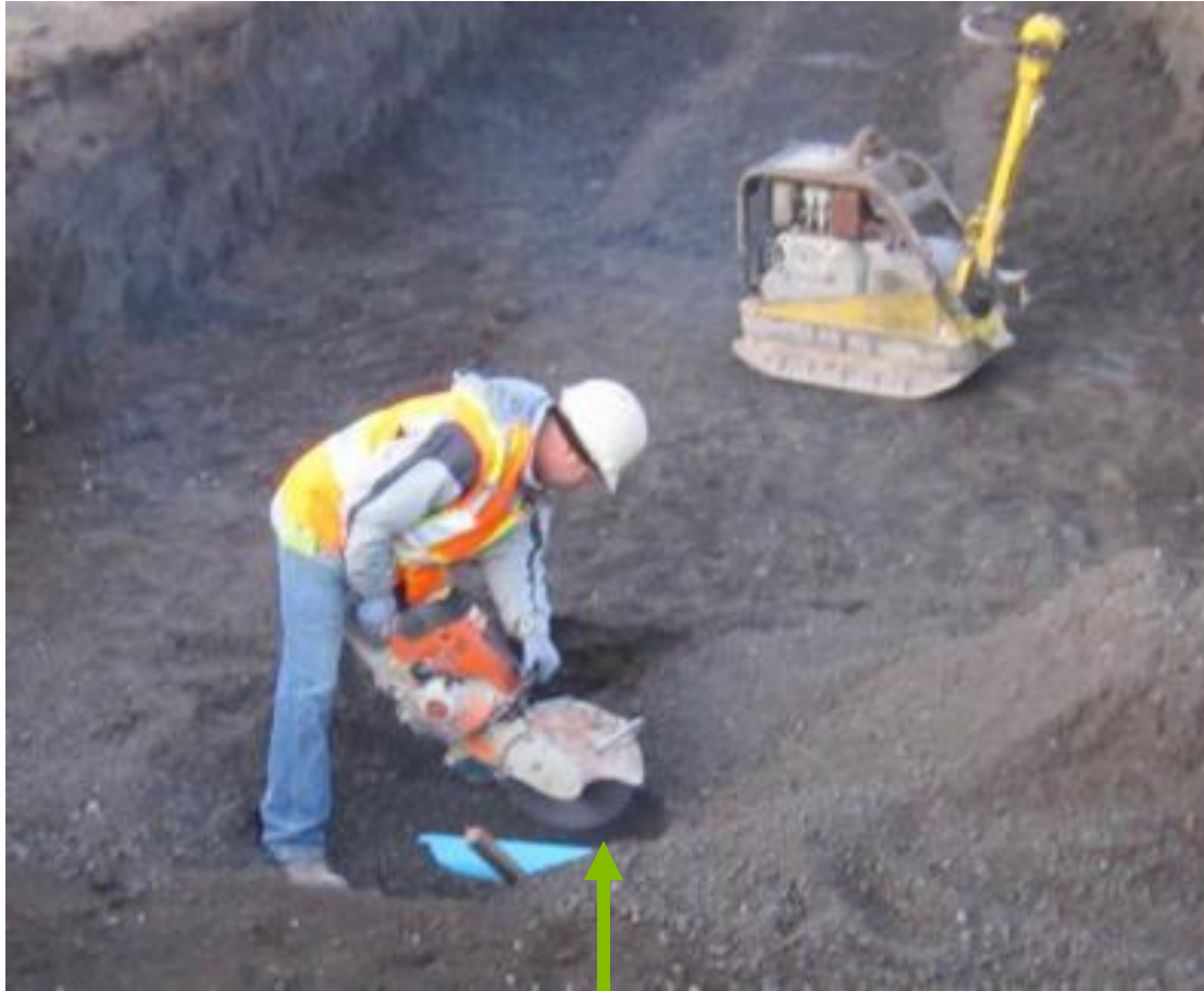
Prior to constructing the Silva Cells, a PVC pipe was buried below the level of the Silva Cells to act as a watermain
