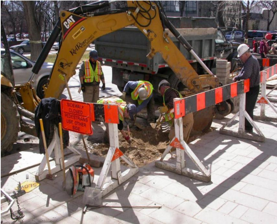
The existing pavement is removed. In this case the existing pavers were salvaged for re -installment
