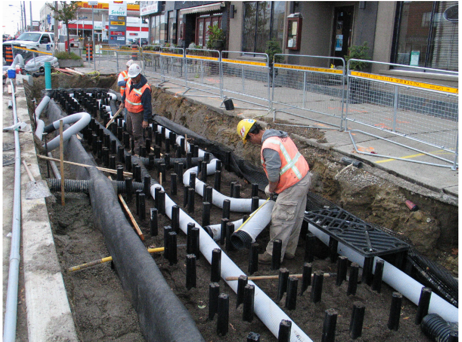
Perforated distribution pipes are placed throughout the system
