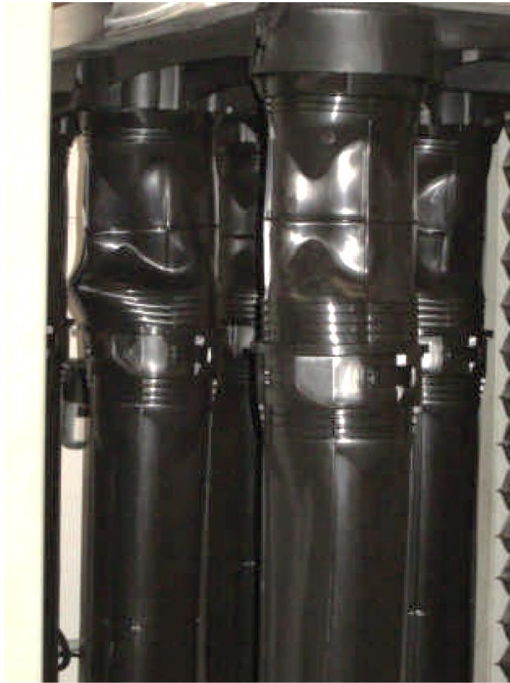
Figure 5: Typical Silva Cell 3X Failure
